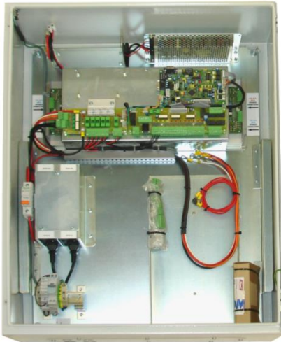
Typical controller cabinet
