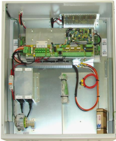
Typical controller cabinet
