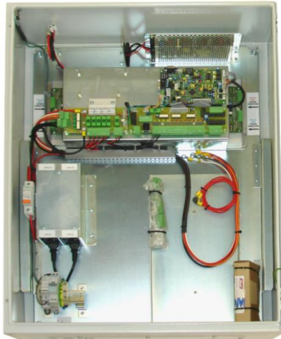
Typical controller cabinet
